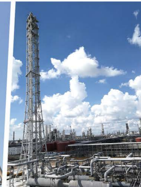
捆绑式高架火炬 (高度 160m, 黑龙江龙油) Multi-stack elevated flare (H=160m, Heilongjiang Longyou)
