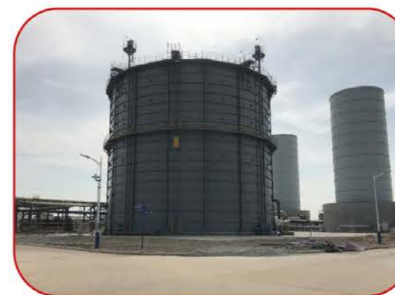
火炬气回收系统 (东莞巨正源) Flare gas recovery system (Dongguan Grand Resource)
