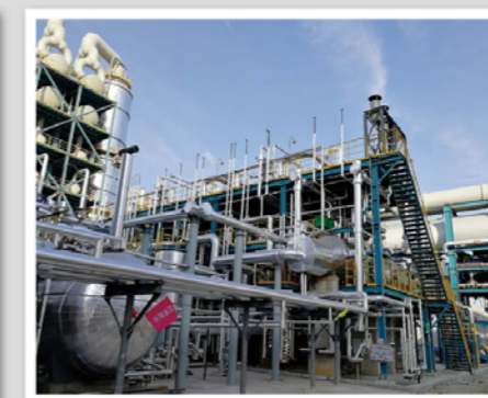
焦化硫回收装置 (日照钢铁) Sulfur recovery unit for Coking (Rizhao Steel)
