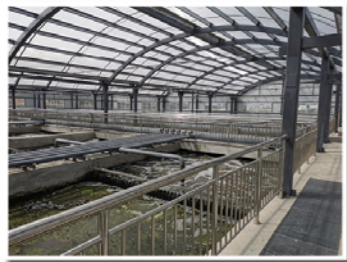
秦安县污水处理厂提标改造工程 Qinan County sewage treatment plant upgrading project
