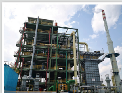
医药废气废液焚烧单元 (台州联化科技) Incineration unit of waste gas and liquid in pharmaceuticals industry (Taizhou Lianhua Technology)
