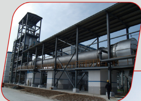
高温回转窑焙烧系统 (神华准能) High temperature rotary kiln roasting system (Shenhua energy)
