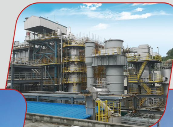
医药危险废物焚烧系统 (华中制药) Hazardous waste incineration system for pharmaceutical industry (Huazhong Pharmacy)
