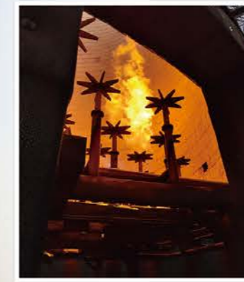
封闭式地面火炬燃烧运行 Enclosed ground flare combustion operation
