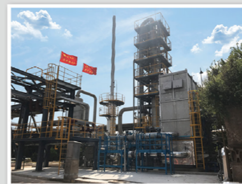
RTO 系统 (上海石化) VOC RTO System (Sinopec Shanghai Petrochemical)
