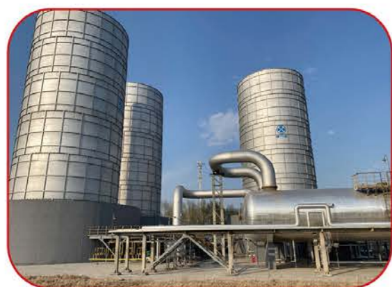
三筒体并联封闭式地面火炬 (吉林康奈尔) Three cylinder parallel enclosed ground flare (Jilin Connell)
