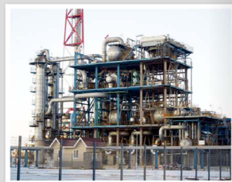
炼化硫回收装置 (辽宁华锦) Sulfur recovery unit for refining and chemical (LiaoningHuajin)
