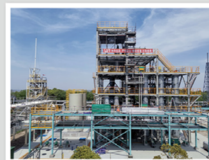
氟化工废气废液焚烧单元 (中化太仓) Incineration unit of waste gas and liquid containing fluorine (SINOCHM Taicang)
