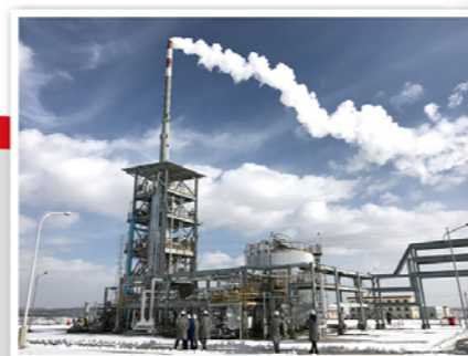
MTO 废碱液焚烧单元 (神华榆林) Quench incineration unit of MTO waste alkali liquor (Shenhua Yulin)
