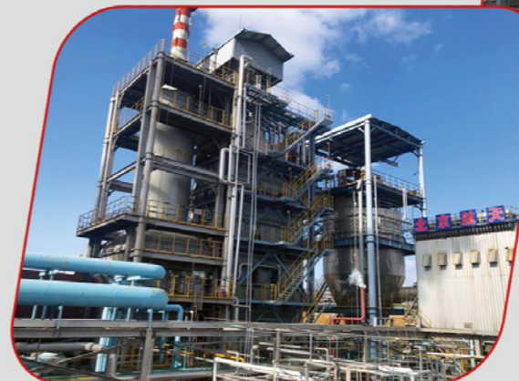
农药危险废物焚烧系统 (江苏辉丰) Hazardous waste incineration system for pesticide industry (Jiangsu Huifeng)
