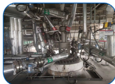
粉煤烧嘴 Pulverized coal burner
